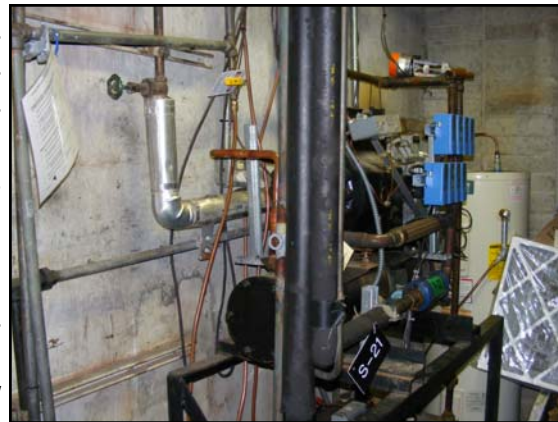
Tesoro water cooled, steam heated air handler
